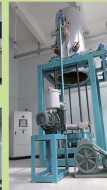
烧结炉 Sintering Furnace
